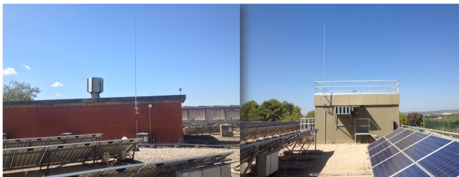
Overview of lightning next to solar panels in drinking water treatment plants
