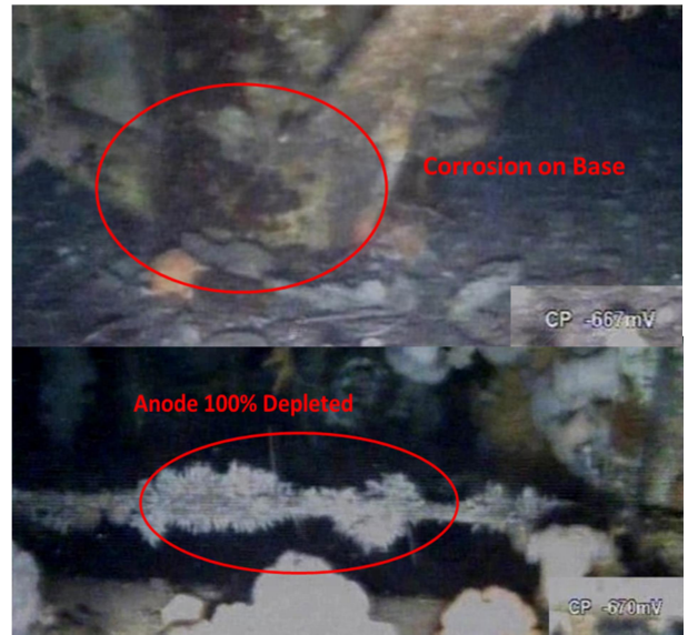
Corrosion on the Protection Frame
